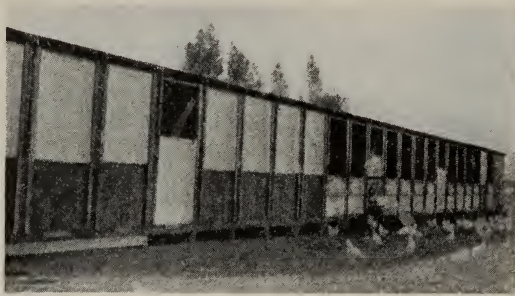
Fig. 12.—Sliding type curtains in use on a poultry house in the Santa Rosa district. Plan for the construction of this curtain shown in figure 13.
